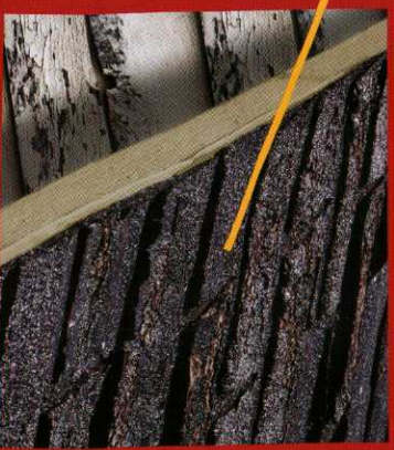
■ Roof shingle, sheathing and siding decay. Possible cause: Poor attic ventilation.
