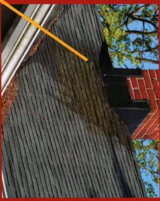
■ Dark, "dirty-looking" areas on your roof. Possible causes: Environmental pollutants, vegetation, fungus or algae growth; loss of granules due to age of shingles.
