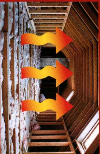
■ Excessive energy costs. Possible cause: Insufficient attic ventilation causes heating/cooling system to run excessively.
