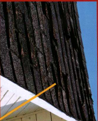
■ Missing, cracked or curling shingles. Possible cause: Shingles have reached the end of their useful life.
